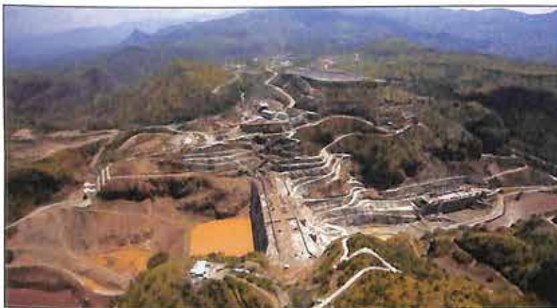
(a) Aerial view of the Gibe III dam site from the right abutment.
