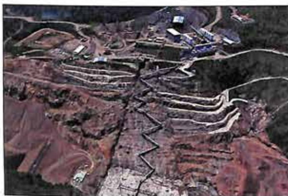
(e) Conveyor belts on the canyon slopes.
