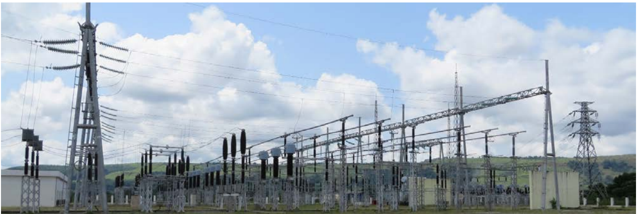
Fig. 5. Existing Moanda 225kV substation with the incoming line from Grand Poubara (SP survey, 2016)
