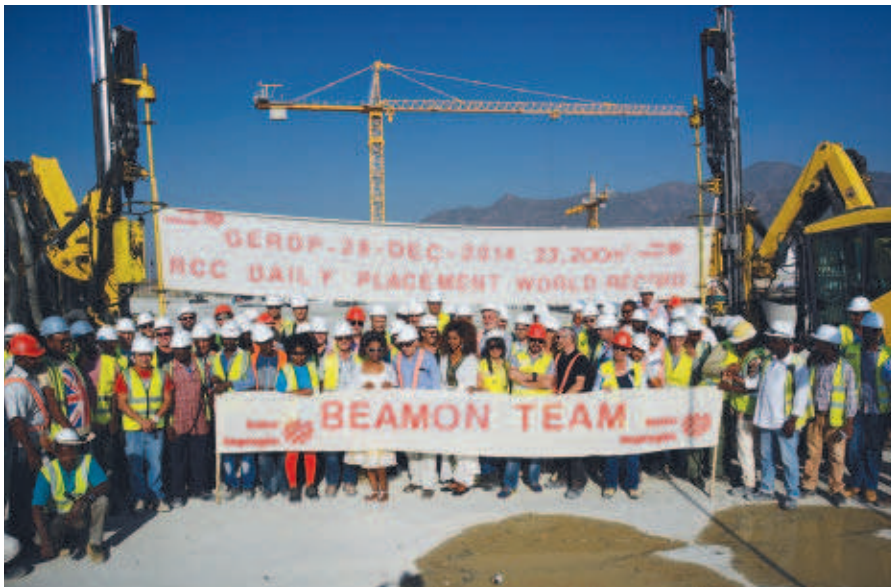
A world record for roller compacted concrete placement was set at the construction site in December 2014, with peaks of 23,200 Mm 3 /day.
