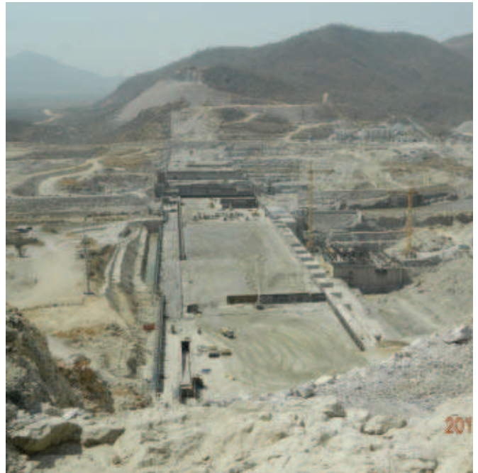
This image, taken on site in January 2015, shows the massive scope of the Grand Ethiopian Renaissance project's Main Dam, photographed from the right abutment.
