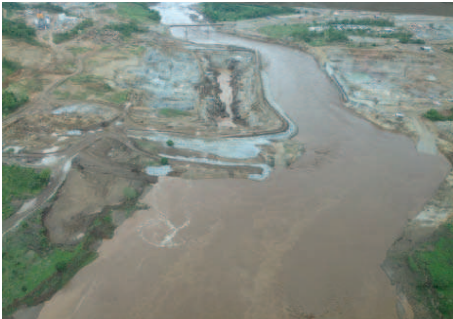
The river diversion scheme changed with the introduction of 2.5 m 3 rock excavation for an additional channel on the right bank, including appurtenant cofferdams and training walls.
