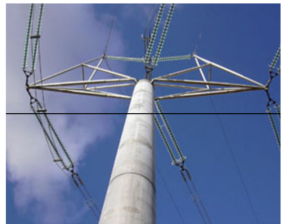
Figure 7 – Angle tower @ BYSTRUP
