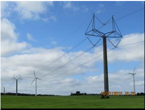
Figure 3 – 400kV line pylon installed in Denmark
