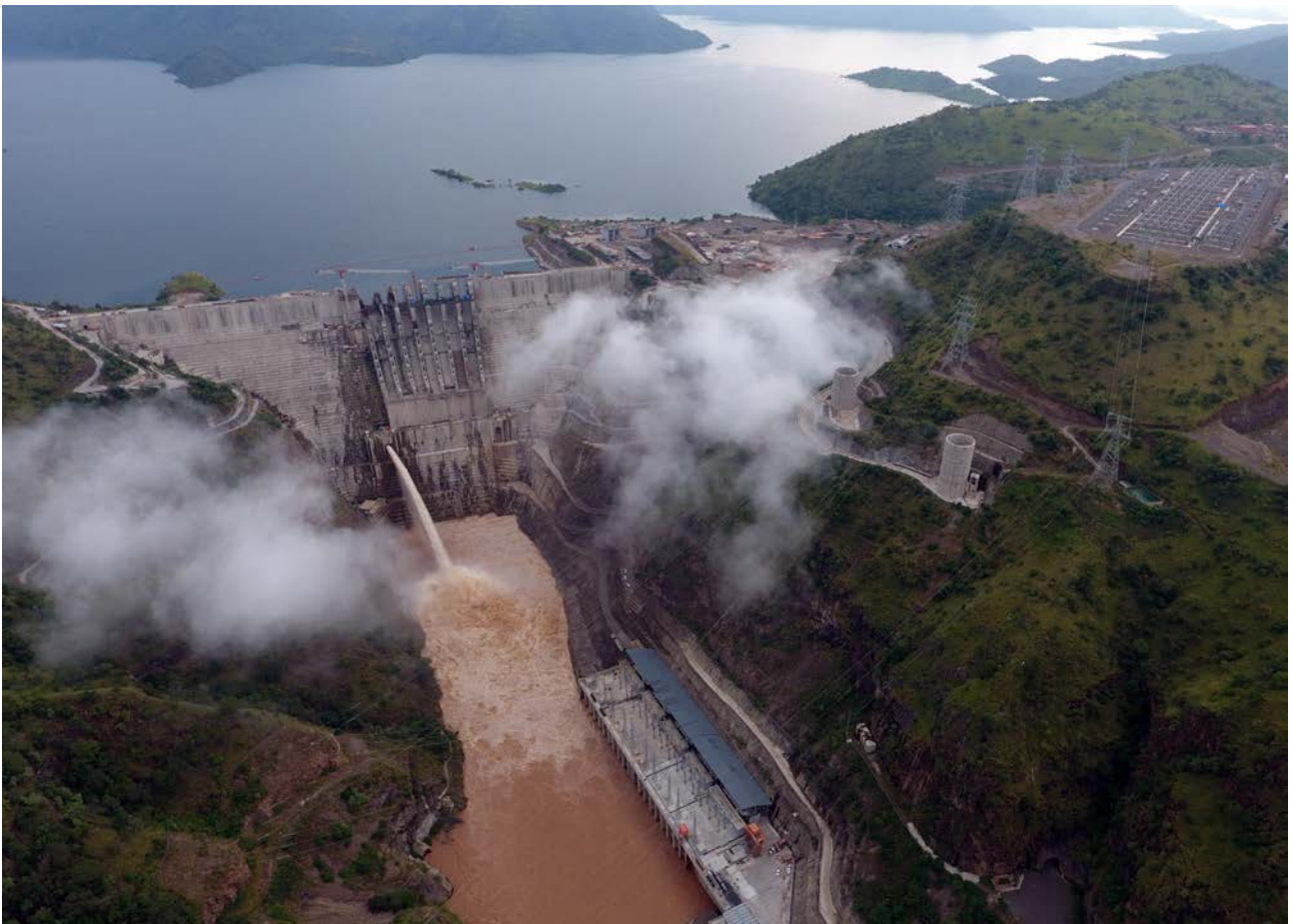
Fig. 1 – View of the dam: spillway under construction, right Middle Level Outlet discharging about 750 m 3 /s (October 2016)
