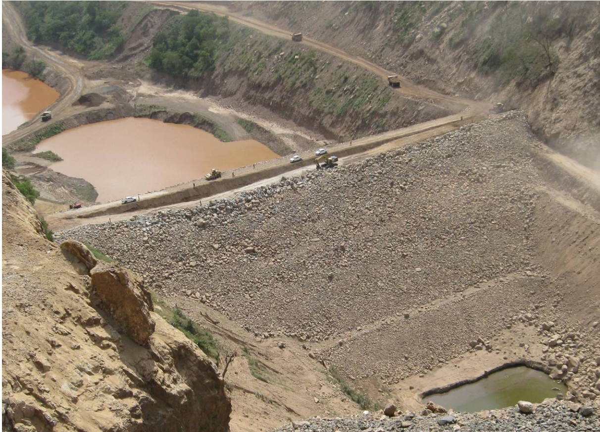
Figure 10. Gibe 3 upstream cofferdam embankment construction completed (on the crest the realization of the crest wall is ongoing)
